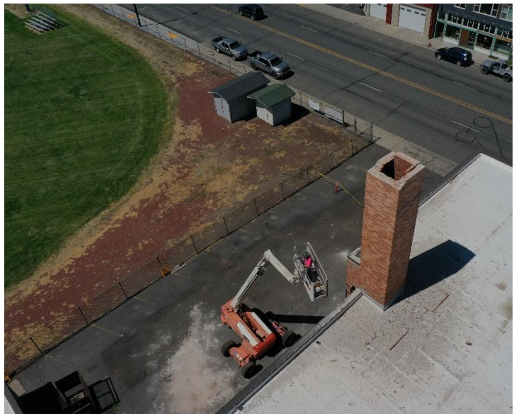
August 16 – Crane day for the Middle School Gym Seismic project. Top photo: crane is ready to lift steel into place. Bottom photo: Unreinforced masonry chimney demolition.
